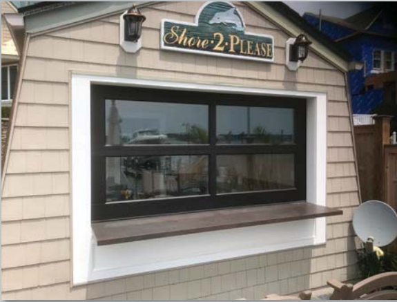
Model MC22-SC Dark Bronze Anodized with Clear Tempered Glass used as a walk up service counter at this seaside snack bar.
